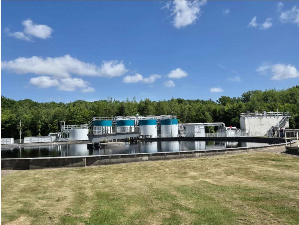
Figura 3 – View of the MicroNutri – O 3 -STEP treatment system at WWTP Winterswijk.
